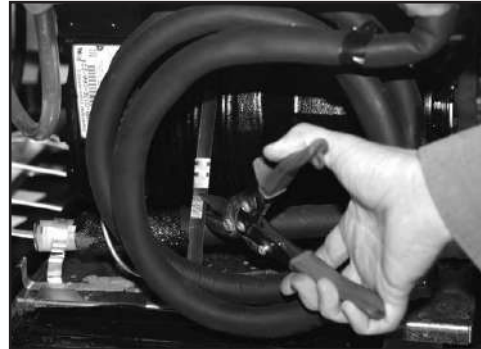
Cutting band that is around compressor
